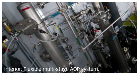
Fully automated control system with data logging.
